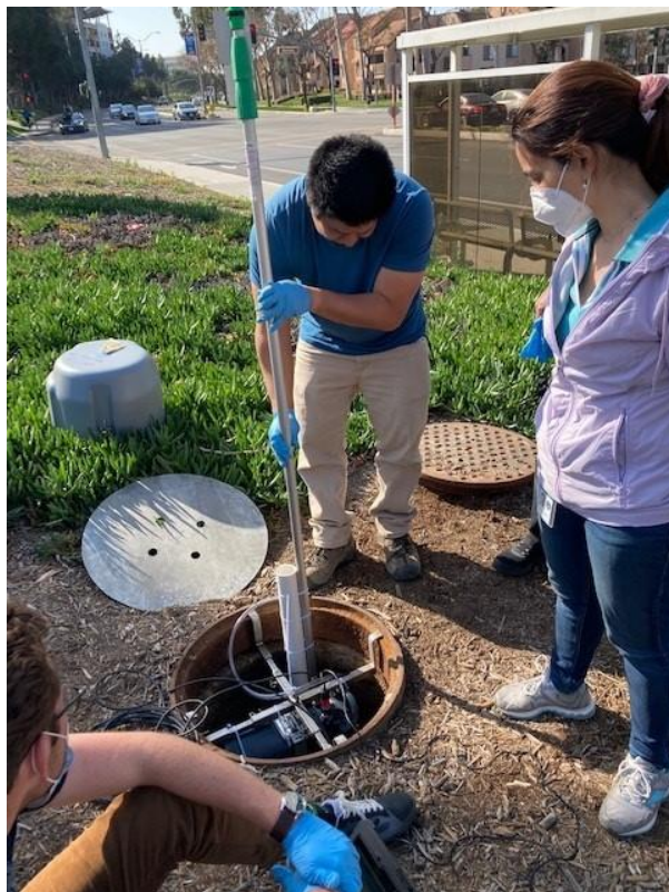
Figure 1 Flow measurement and sewage sampling device installation at a sewer manhole near UCI campus. June 2022
